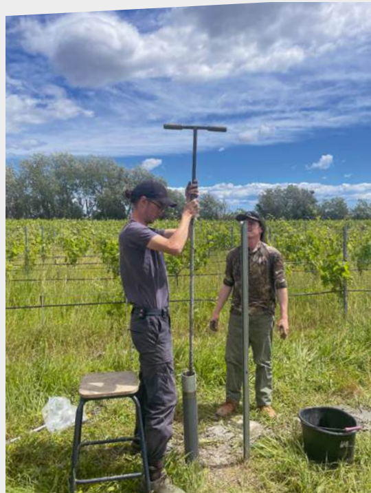
Installation of a piezometer in vineyard plots affected by salinisation, carried out by Morgan Garnodon and Django De Herder.
